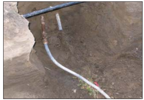
After a typical partial lead service line replacement, new copper pipe is connected to the remaining lead service line. The pipe running slantwise across the top of the photo marks the border of the property line. The pipe on the right is the lead service line left in the ground. The connection on the left shows the new copper pipe (short segment) attached to the remaining lead service line.
